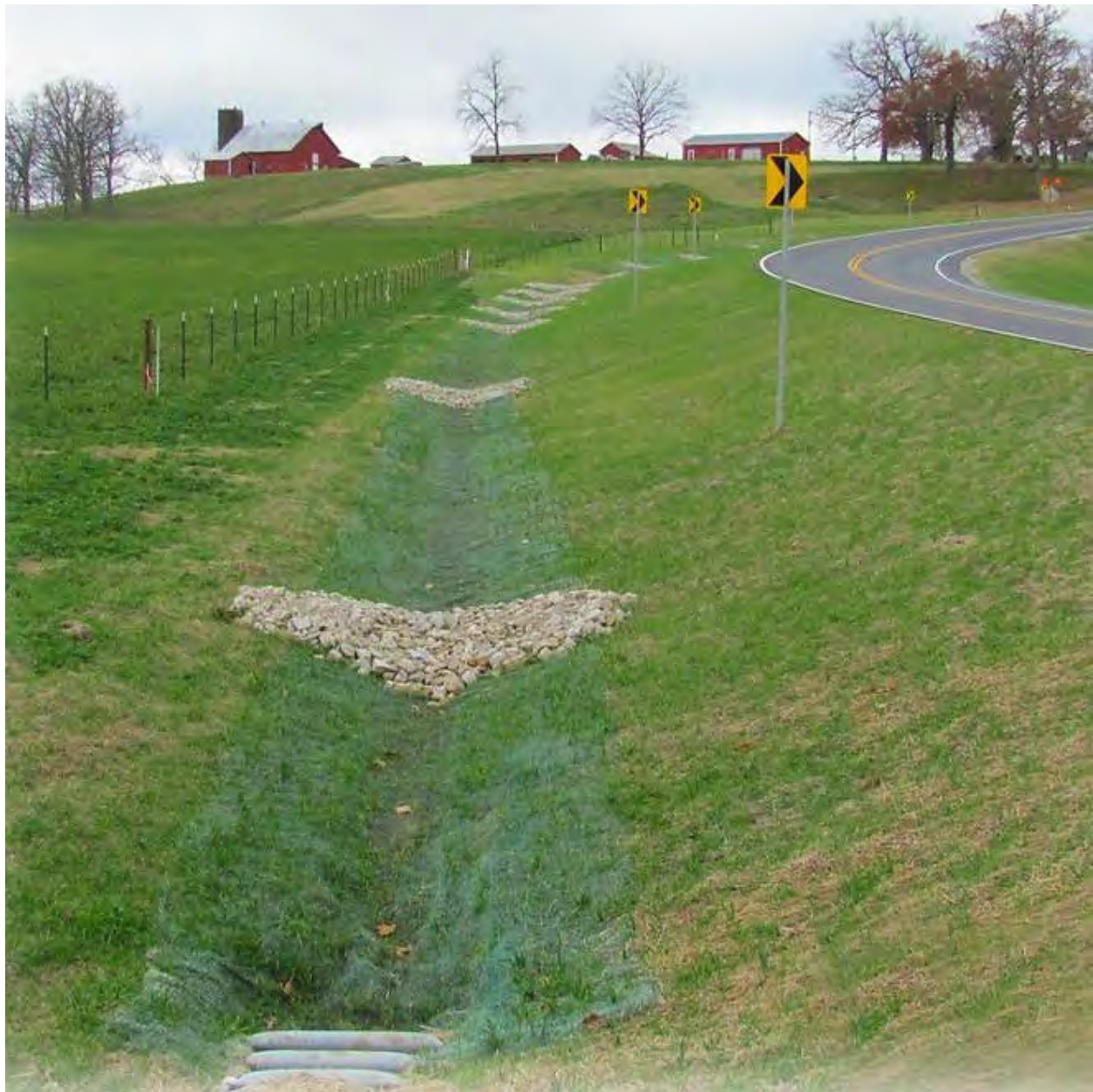
Figure 58 – Rip-Rap Check Dams in Roadside Swales
